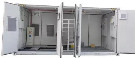
1075KW HH ESS
