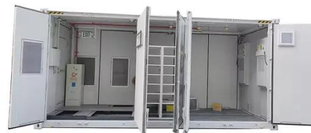
1075KW HH ESS
