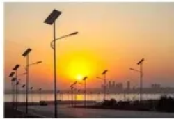
Solar Street Light
