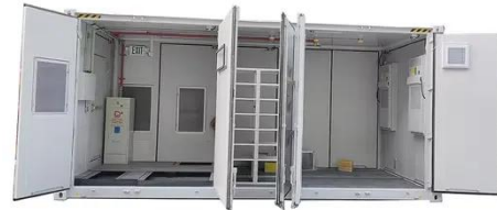
1075KW HH ESS
