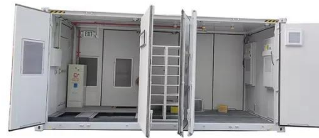
1075KW HH ESS
