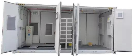
1075KW HH ESS
