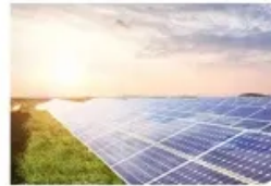
Energy Storage System
